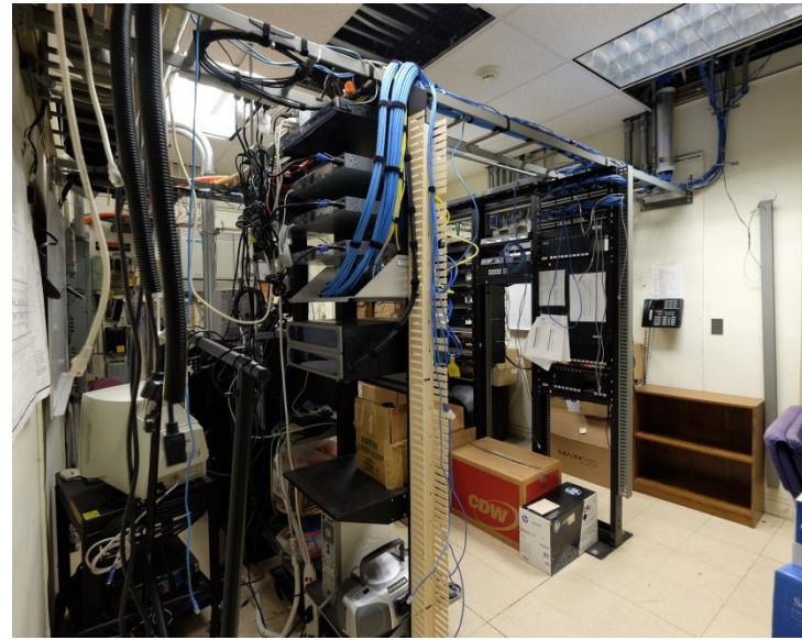
Photo 9 Building Name: Admin/Classroom Building Building Number: 1 Electrical room
