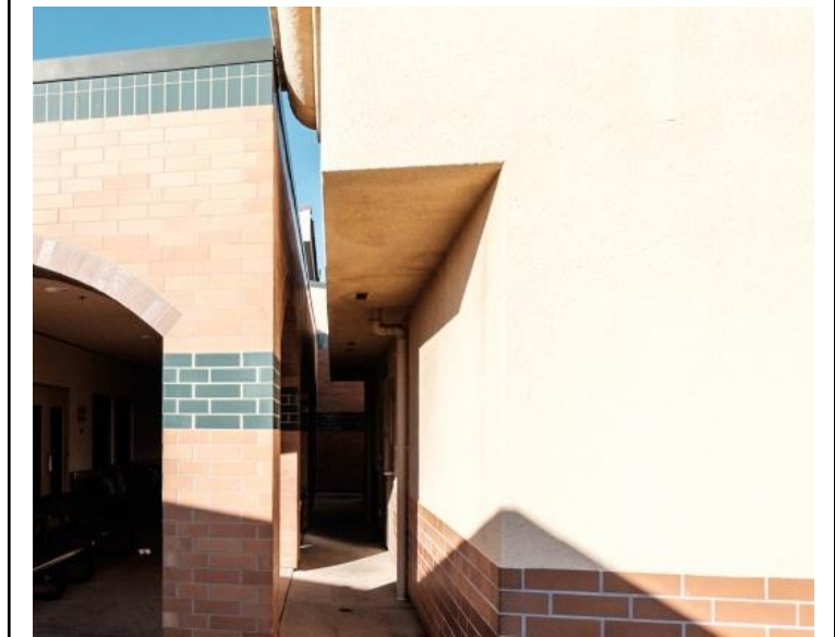
Photo 24 Building Name: Classroom Building (Modular) Building Number: 3 Building 1 and Building 3 touching at parapet and tight space between buildings.
