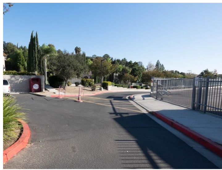
Photo -1 Pedestrian entrance from Knightsbridge Avenue. There's a security issue because a permanent gate was not installed to control access.
